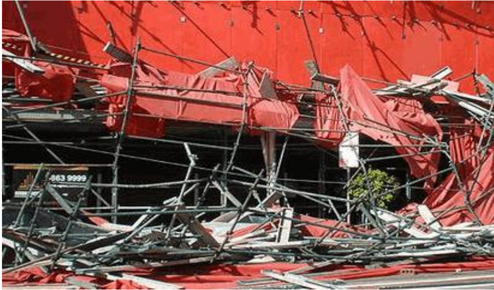
MELBOURNE - Prahran scaffolding collapse - February 24th, 2009
