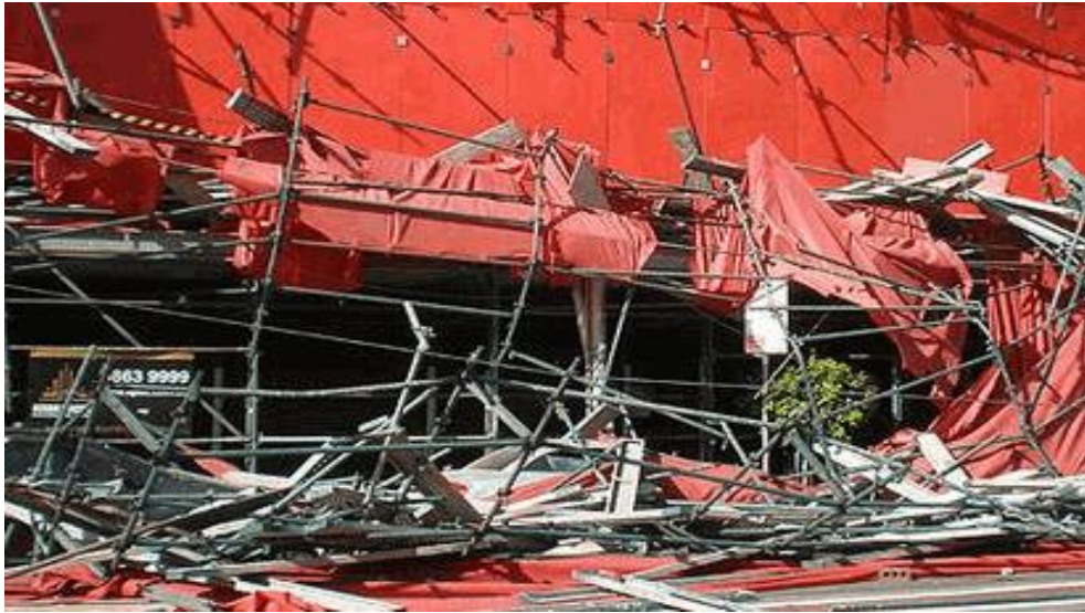
MELBOURNE - Prahran scaffolding collapse - February 24th, 2009
